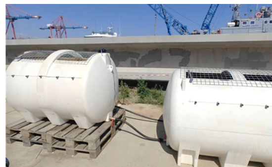
4: Open-air algal pilot installation.
